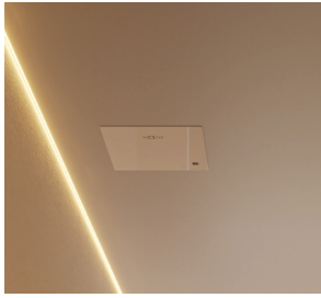
Recessed in ceiling
